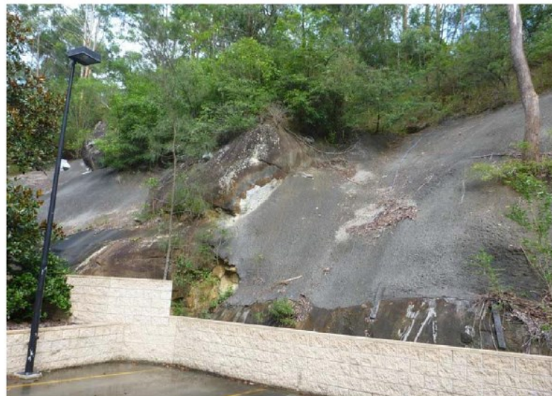
Photo 6 - Unsupported slope above shotcrete face in Area 3
